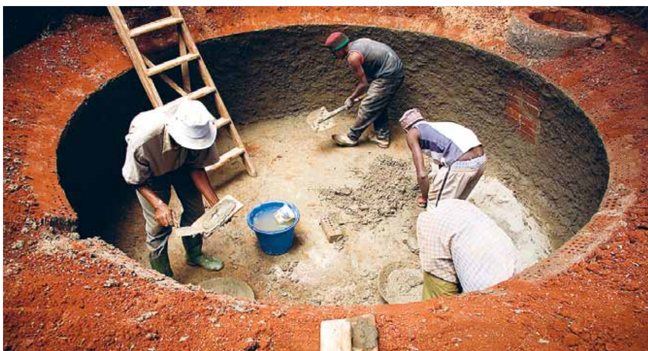
Men at work on a Biogas project, which was supported by the Rosminian Fathers. This project has benefited a local community outside Ngong town in Kenya. Photo: Amy Colley.
